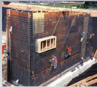
Advanced Micro Devices Fab 25 Industrial Water and Acid Waste Building 110,000 Sq. Ft.
