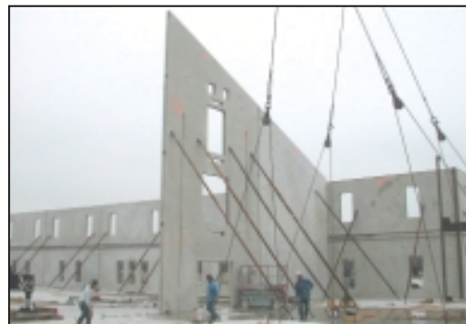
The raising of tiltwall panels at the new high school for Leander Independent School District in Cedar Park.
