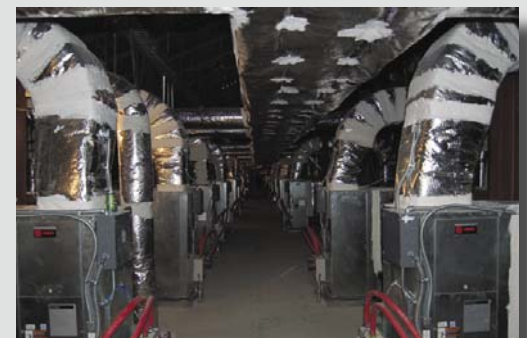
In this school, air conditioning units were relocated from individual classrooms to a mezzanine above, resulting in quieter classrooms and equipment in a location where it was easier to service.
