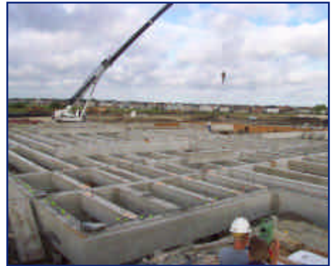
American Constructor's precast yard for the RRISD Stadium Complex where nearly 400 concrete beams were cast to precise specifications.
